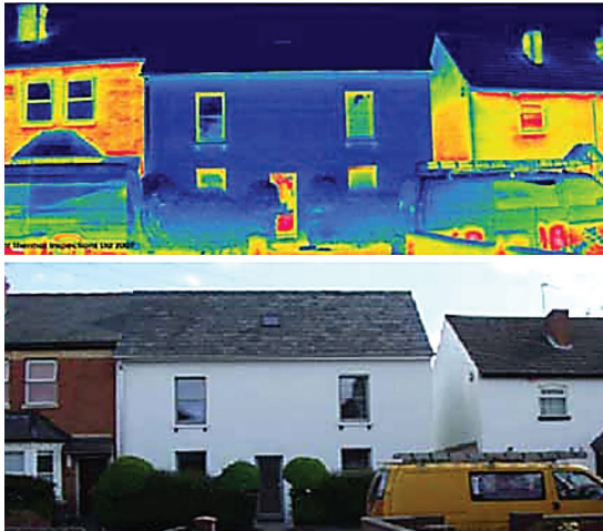
©Grove Cottage (c) Sirmmonds,Mills / Thermal Inspections Ltd
